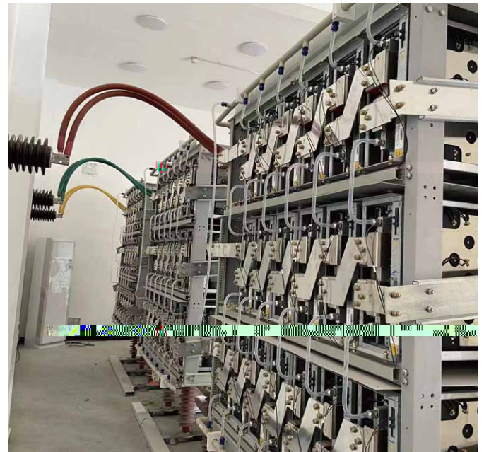
Water cooling system
